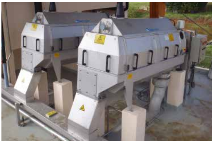
Roto-Sieve drum screens, model RS-24, installed at Guadeloupe treatment plant for the protection of plant membranes.
