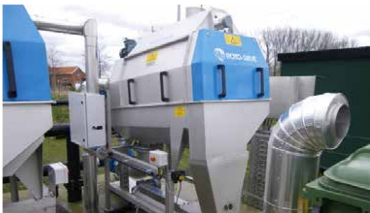
Roto-Sieve drum screens, model RS-22, installed at Zwalm treatment plant for the protection of plant membranes.
